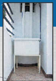
External split unit
